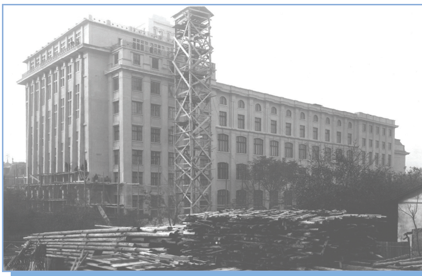
Erecting the Lecture Theatre Building (view from the current Stanislas Cihoski Street)
